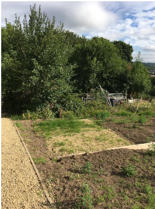
Cleared and prepared allotment plot with new base to accept Council provided shed or greenhouse
